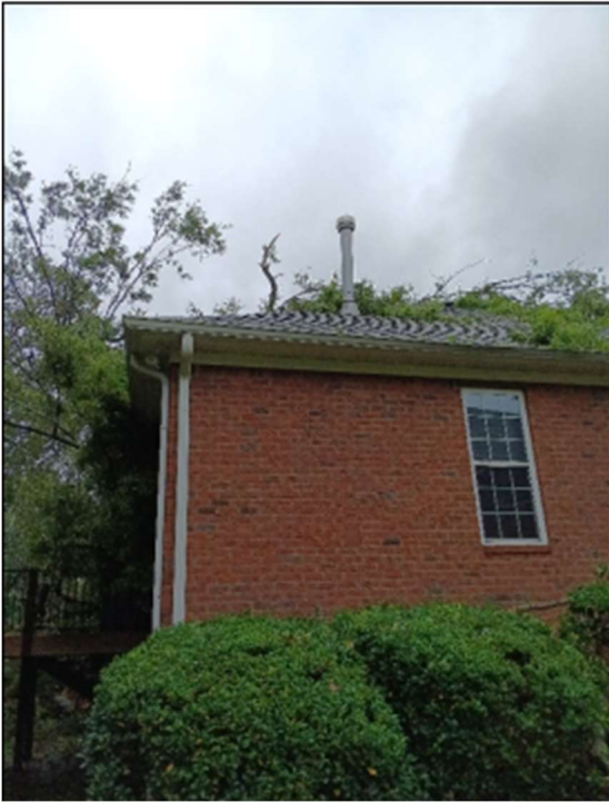
Holes above Katherine's room and Scott's office:
