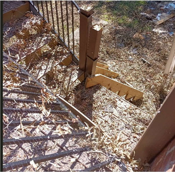
Stairs gone! Railing crushed on the side.
